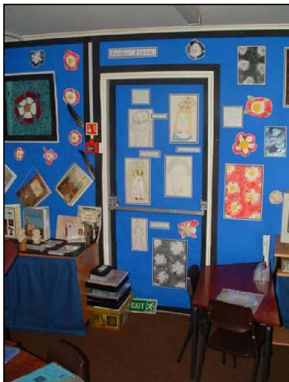
Fire exit door is covered in a display so not clearly visible, fire exit sign is propped up by the door and boxes are blocking the exit.
